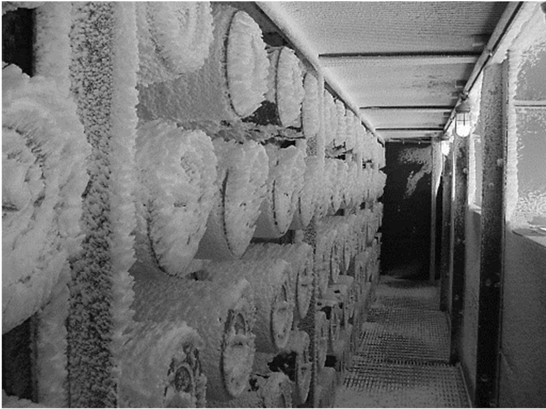
Figure F.19—Horizontal Cartridge Filters with Frost Buildup Due to Cooling Tower Drift
