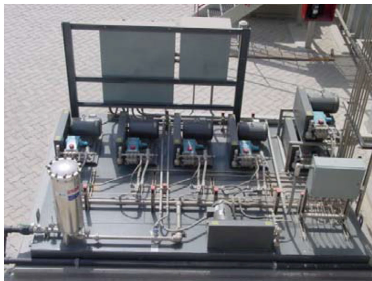
Figure G.5—Typical High-pressure Fogging Skid
