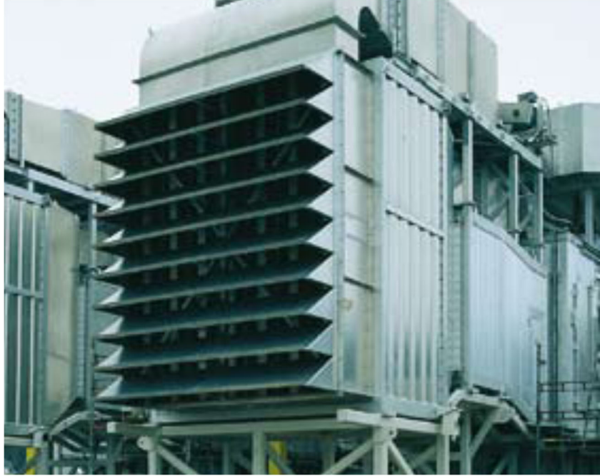
Figure F.18—Weather Hood on Inlet Air Filtration System
